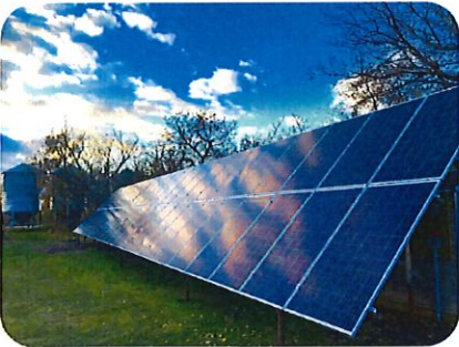
15.6 kW solar system
