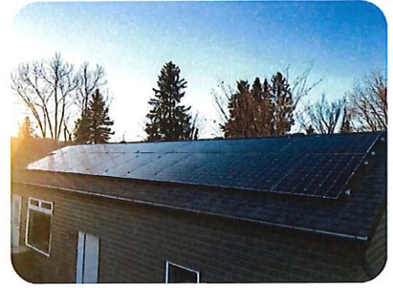
6.4 kW solar system
