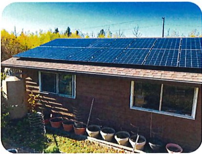
5.5 kW solar system
