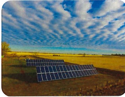
26 kW solar system
