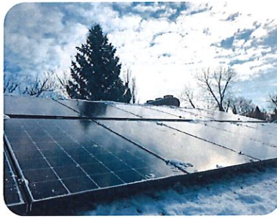
8.0 kW solar system
